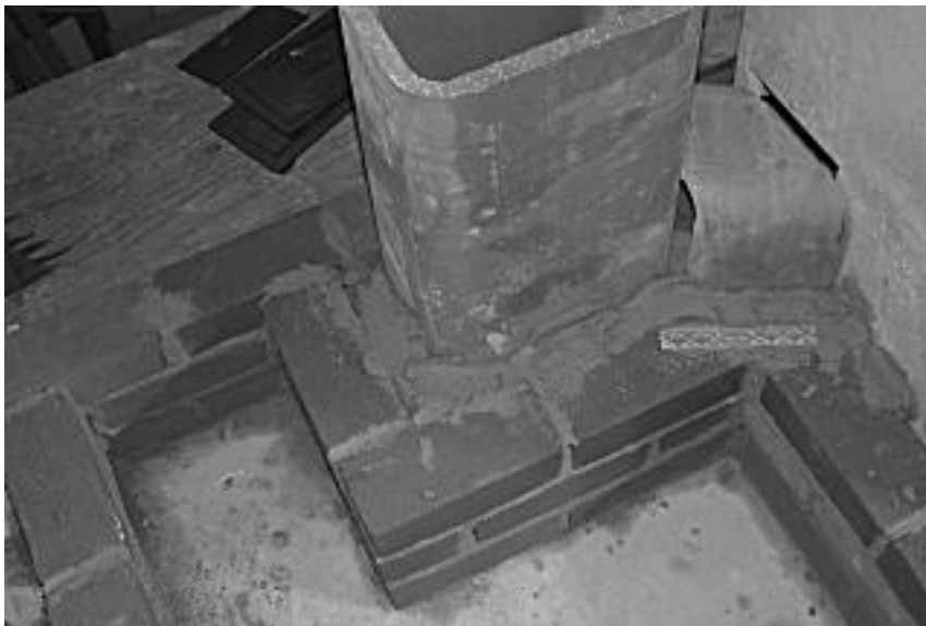
Figure 5. Mortar slush around flue liners.
